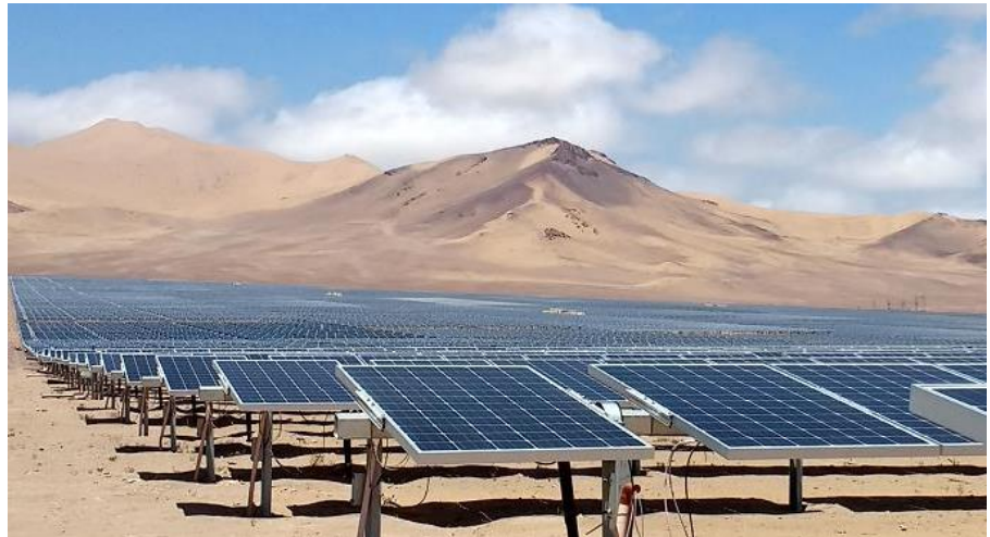
Figure 2: Benban solar park
